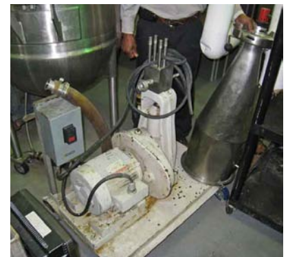
Feed Pump Fines Cyclone
