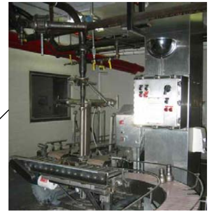
Discharge & Control Panels
