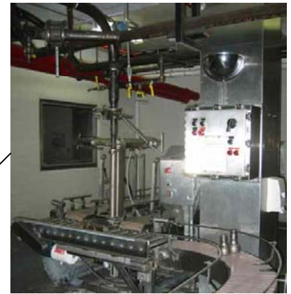
Discharge & Control Panels
